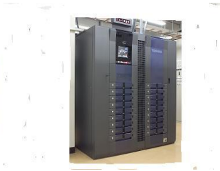
3 kW digital transmitter rack
